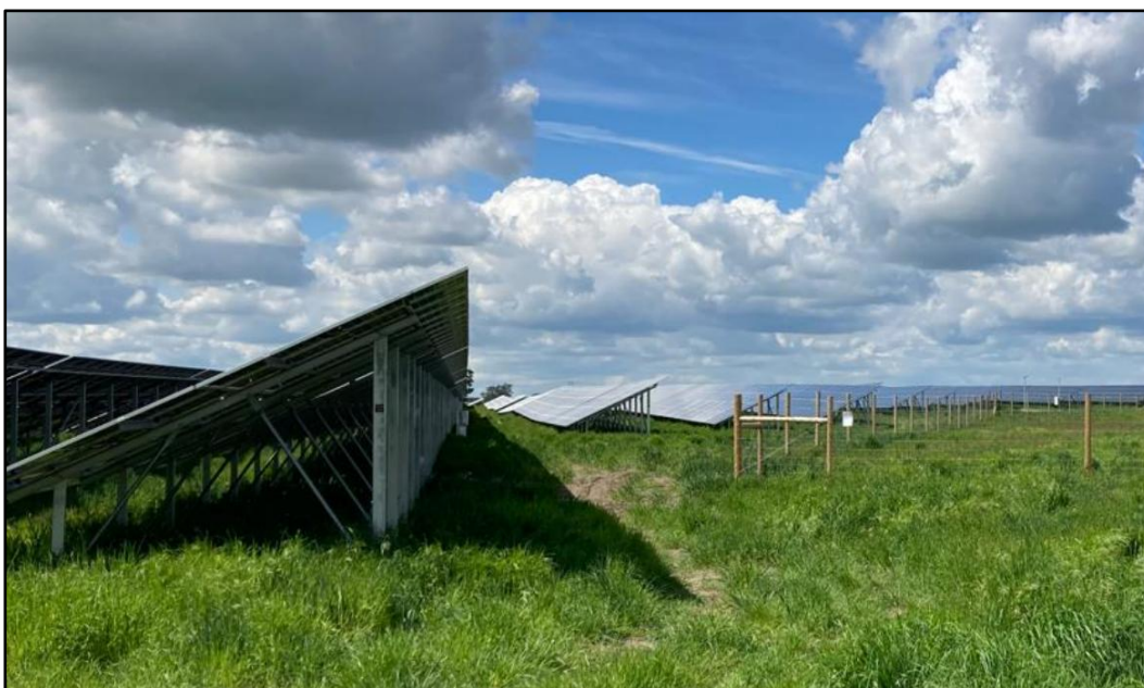
Plate 3.2 Example of a typical mounting structure
